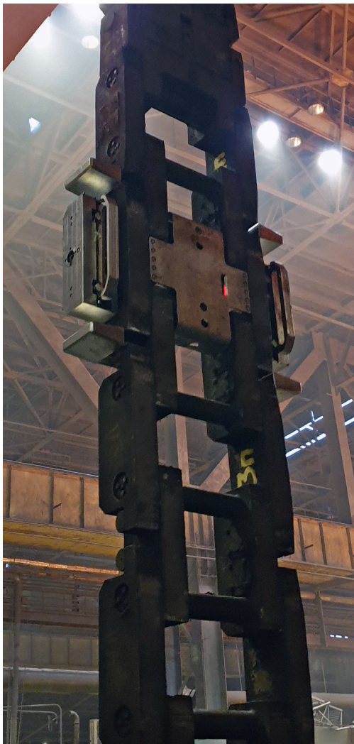
The images shown are the completed installation. The top image shows the dummy bar chain in its home position and battery charging cable connected.
